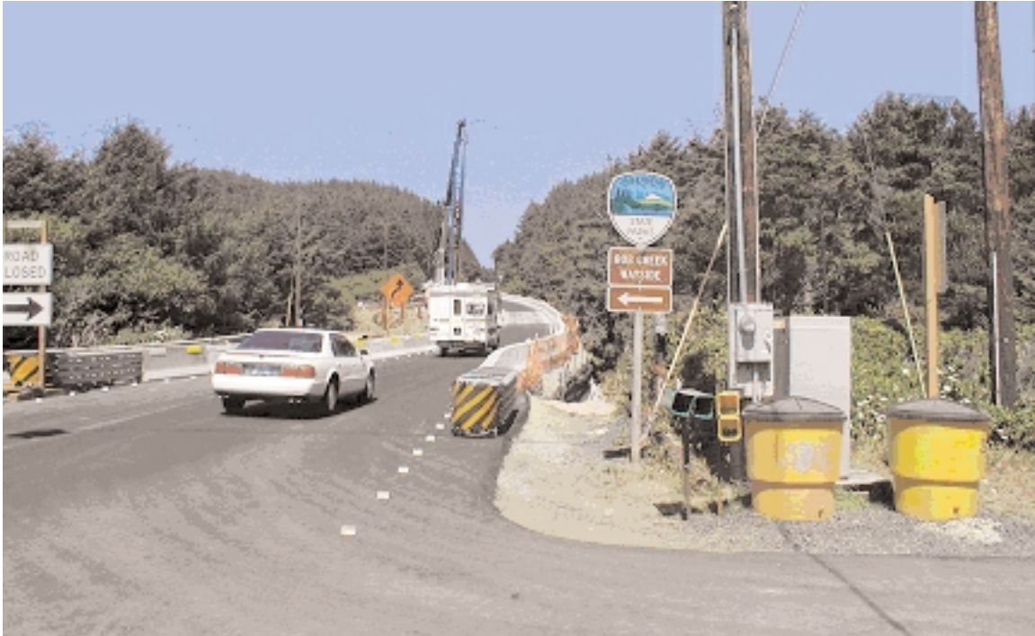
Diverted traffic used the MSE bridge while the permanent Bob Creek Bridge was being rebuilt.
